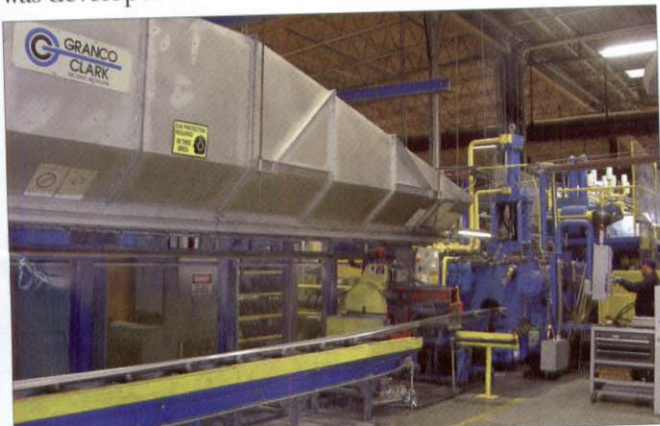
Figure 2. Pictured in the foreground downstream of the 7" BLH press is a Granco Clark quench system.
